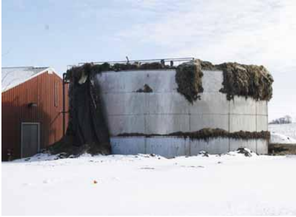
Waste treatment tank at Cavel ruptures and foams over, March 2007.
